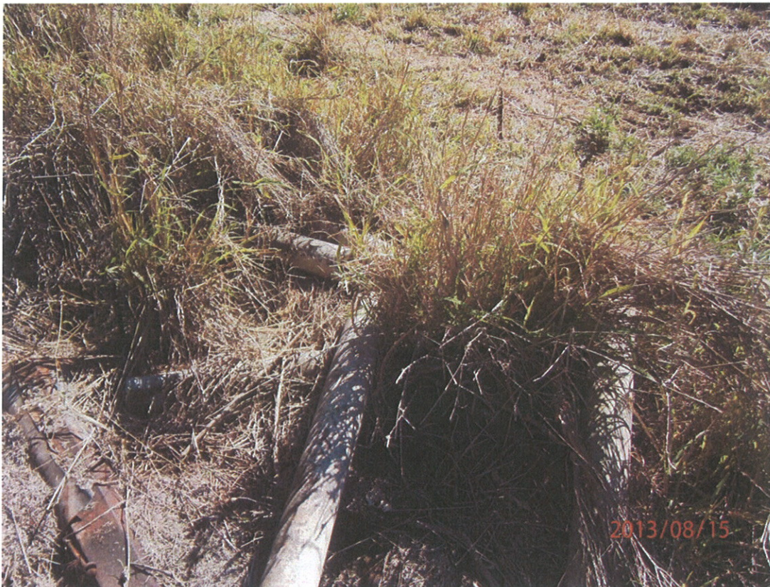
Photograph 4 – Suspected asbestos containing material (ACM) pipe
